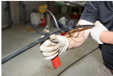
Peel the sheath off the steel wires along the entire length to be peeled.
