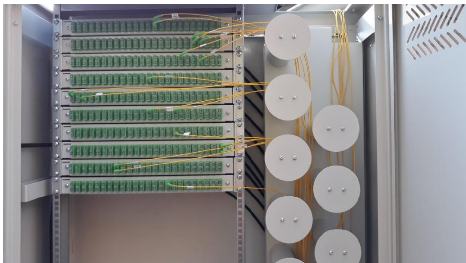
The patch cords going out of the XC-cabinet to the equipment cabinet.
