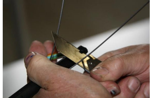
Thin the ends of the cable a little. Thus, they go more easily through the cable glands, but this is also necessary for the installation of earthing connectors.
